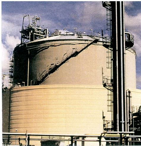
Fig.11 LNG storage tank and bund wall. (Courtesy of BG Storage)
