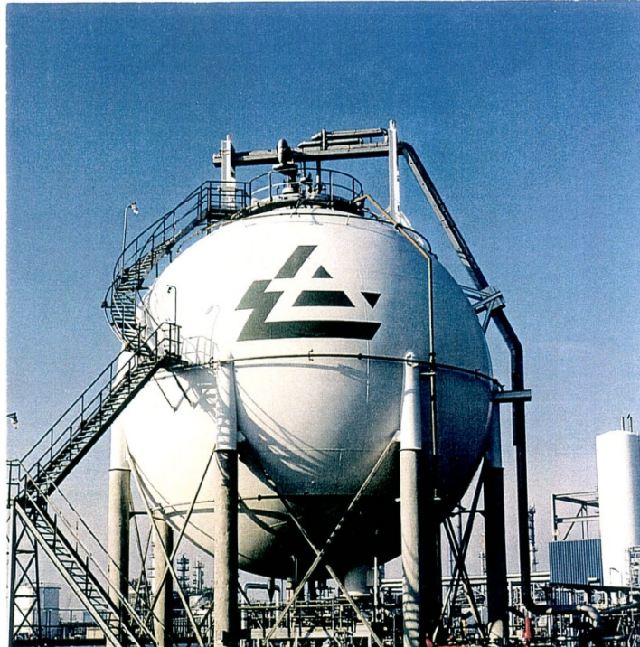
Fig.12 Liquid hydrogen storage tank (Courtesy Air Products)
