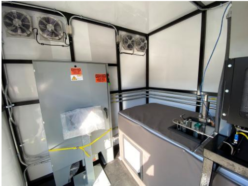
Additional HMI on Pedestal
