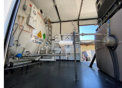
Clear Space Avoiding Trip Hazards
