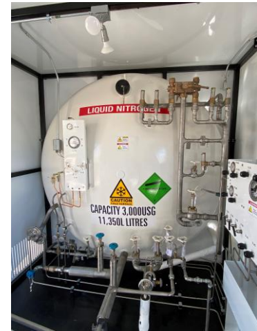
Valve Cluster for Fill and Prime
